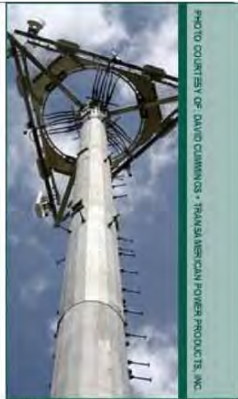
Platform mounted, sectorized, cellular telephone antennas. The fat monopole depicted is necessary to hold the platform.
