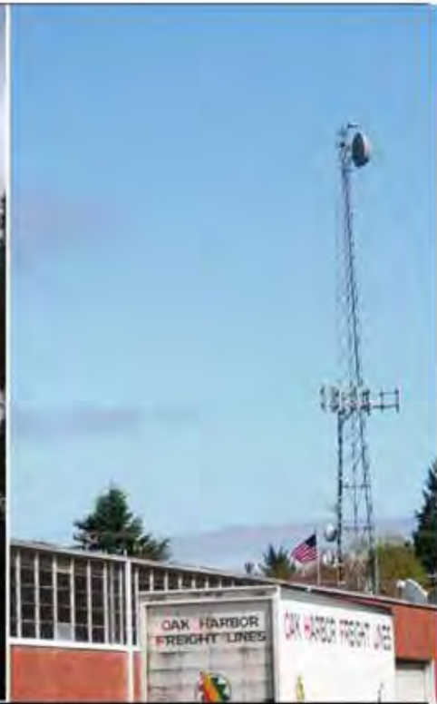
A-frame lattice tower with one microwave link and one carrier
