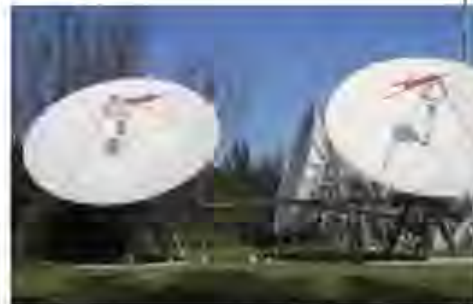
Cable TV headend with several dishes and tower
