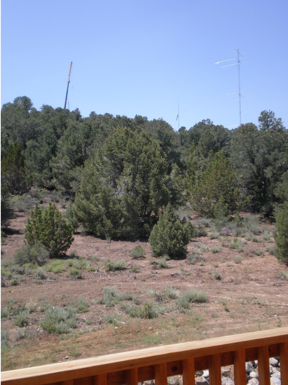
Exhibit E: Crane working away on tower #1 – doubling the size after being warned the day before that a SUP would be required.
