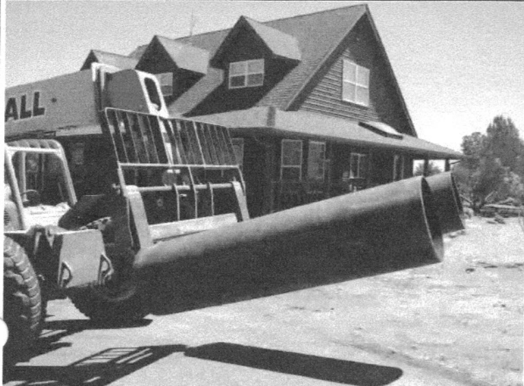
The bases for the 140' and 200' rotating monopoles are 20" OD, 19" ID Pipe 7.5' long. They will be placed in a 5' hole with rebar and concrete inside and out.
